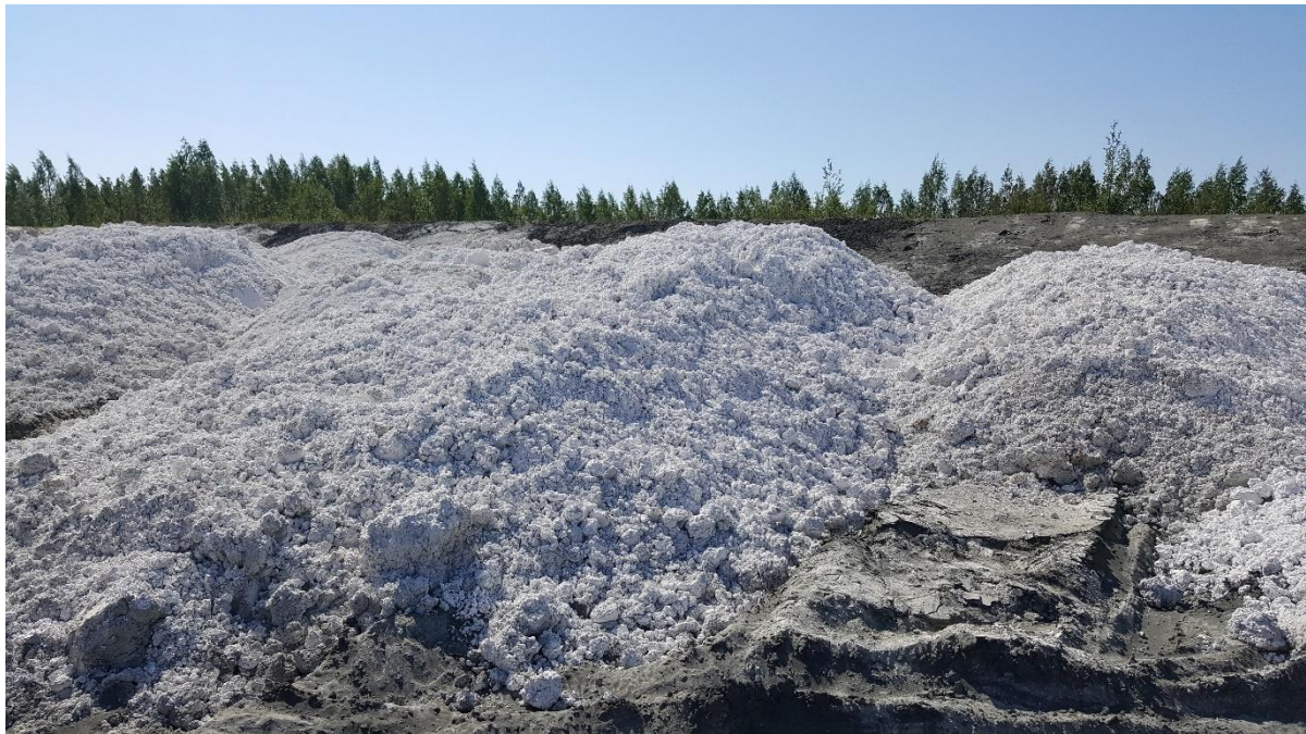
Figure 4. Fibre clay in Hitura construction site before used in the piloting structure.
