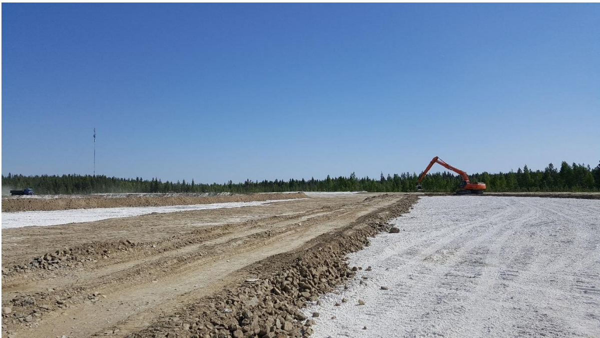
Figure 6. Fibre clay utilisation in Hitura did not require any special vehicle or equipment.
